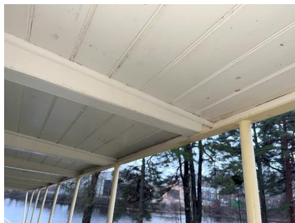
Himling, takoverbygning – dekk. Feste septe, bjelkelag himling.
