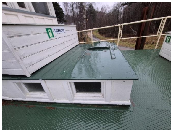
Lysventiler, casing forut, styrbod side.
